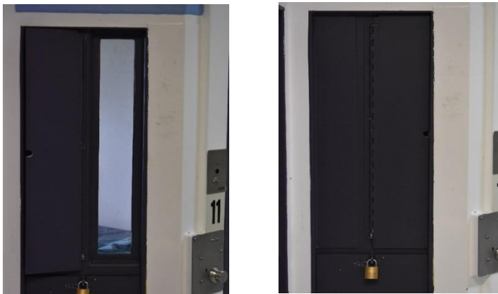
Images of metal shutters on the outside of viewing windows in at-risk cells
